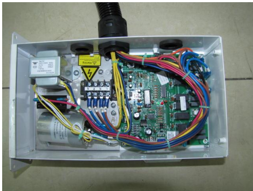
Electric box internal view
