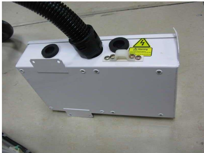
Electrical box view
