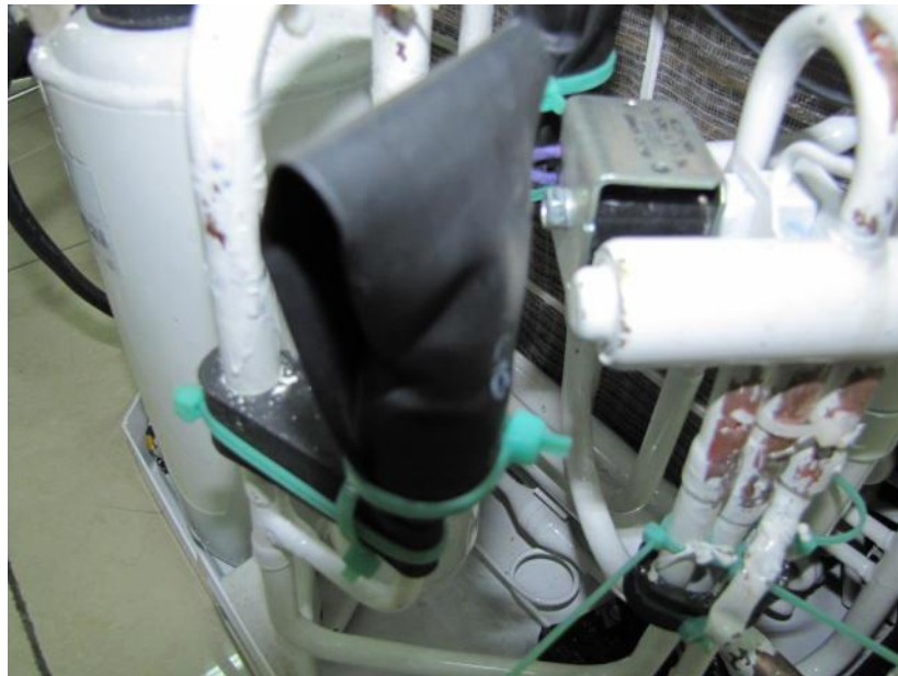
All pressure switch were wrapped
