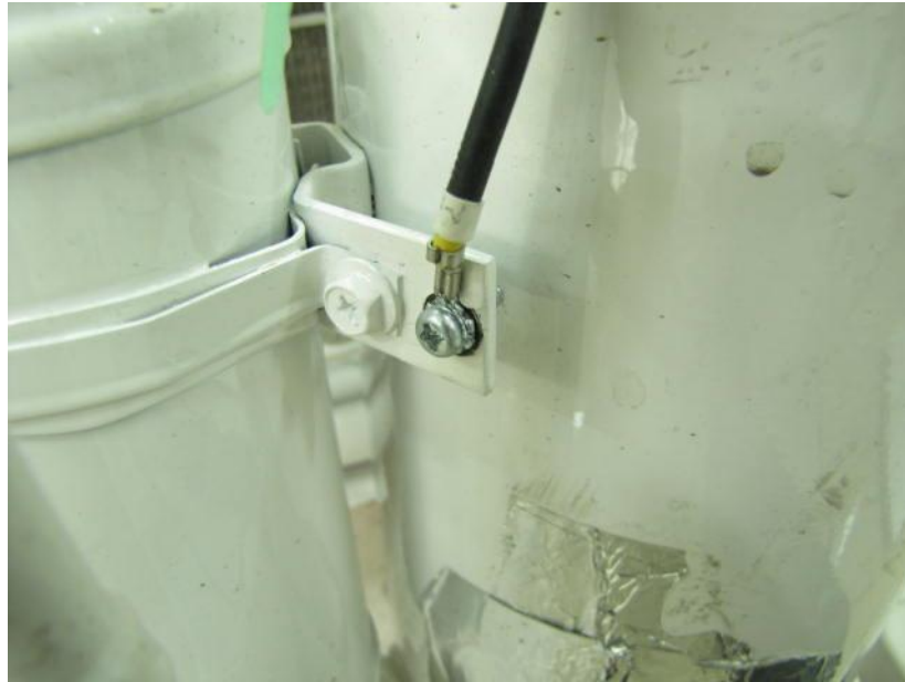
Compressor earthing view
