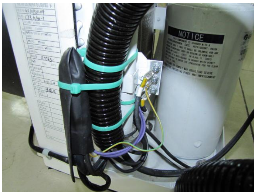
Wireway and compressor view
