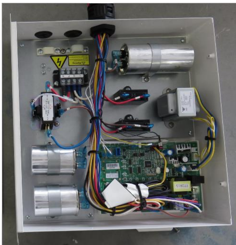
Main power box
