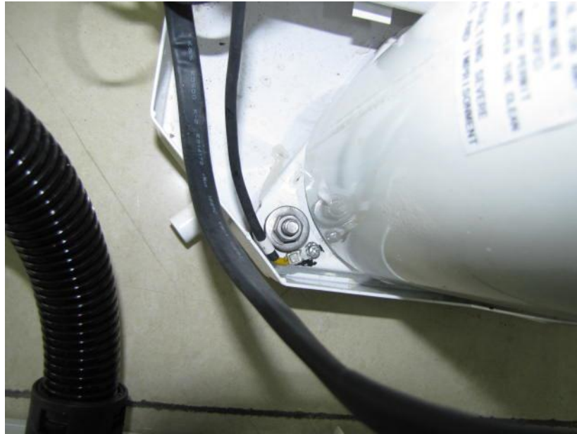
Compressor earthing view
