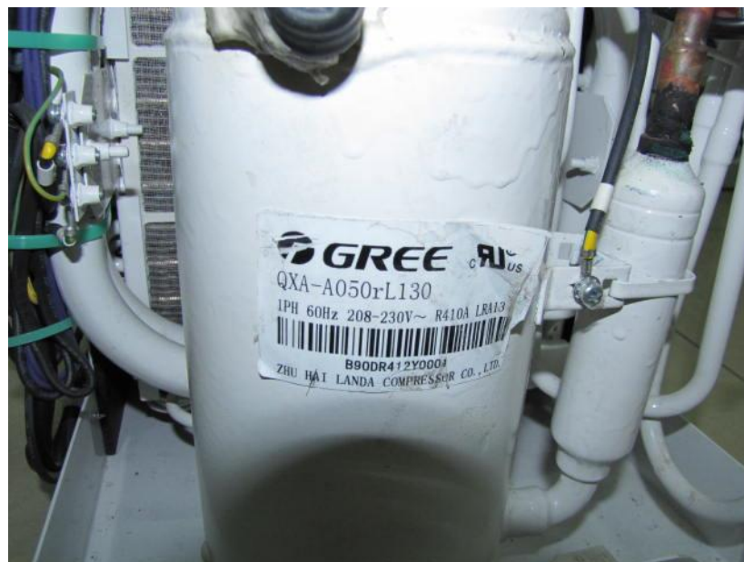
Compressor and earthing view
